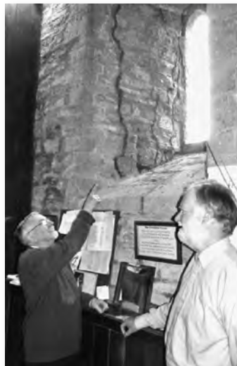
St. Kenelm's PCC treasurer Bob Davies points to the cracks that have appeared in the church tower following water damage.
